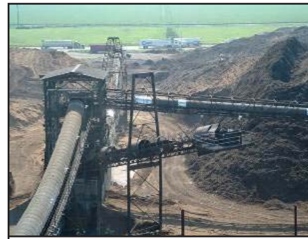
Okeelanta Co-generation facility burns woody biomass and sugarcane waste.
